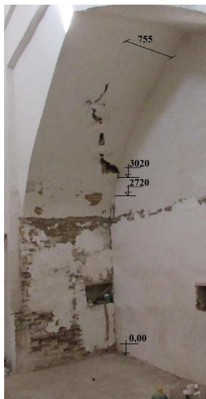
7-picture. The size of the cracks that appeared on the wall on the north side of the large room was determined
