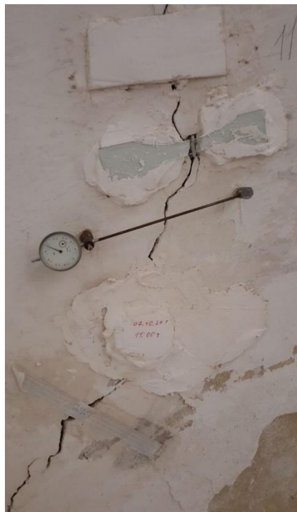
6-picture. A clock-Type Indicator was installed on the cracks that appeared on the wall of the large room
